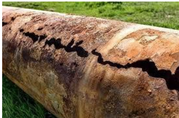
Figure 0.1: Erosion corroded metallic component (Source: ((Ajoku et al., 2021))
