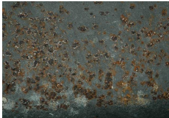
Figure 0.4: Image showing pitting corrosion ( https://steelfabservices.com.au/pitting-corrosion/ )
