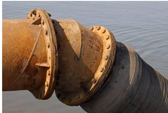
Figure 0.7: Image showing atmospheric corrosion (Source: Ajoku et al., 2021).
