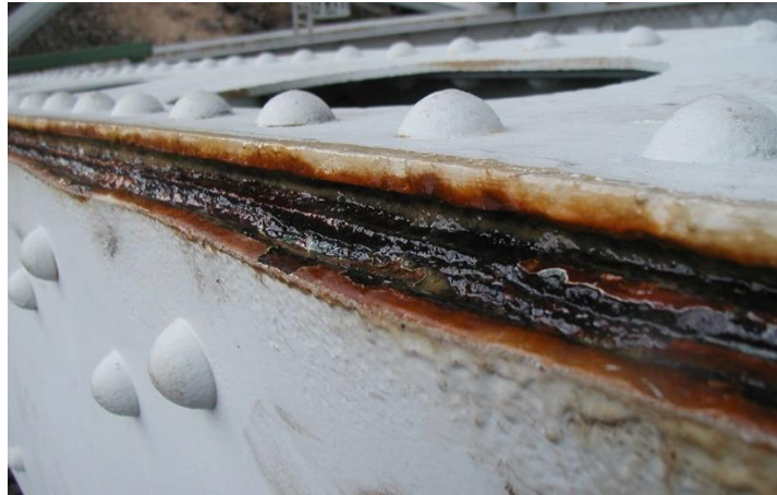
Figure 0.5: Image showing crevice corrosion ( https://steelfabservices.com.au/crevice-corrosion/ )
