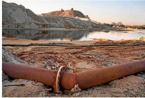
Figure 1.4: Oxidation wear on pipes from Grootvlei mine plants (Adopted from Mukhuthu, 2014)
