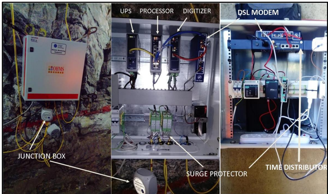
691 692 Figure 3.6: Underground seismological monitoring equipment set up.
