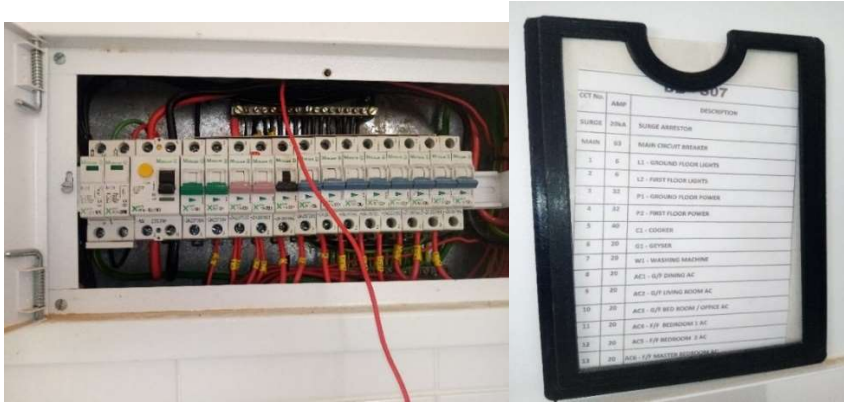
Figure 3.4: The distribution board (DB) of the house in the experiment and electrical appliances list.
