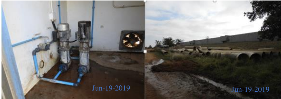
Figure 5. Water leakages on a chlorination plant located in Foresthill (Kgale) (left) and losses through water pipes located at Diremogolo reservoir, Gabane (right).
