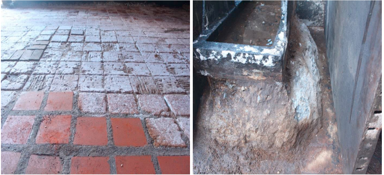
Fig. 1. Corrosion effects of Ammonium Nitrate on (a) plant floors (b) concrete bases supporting heavy machinery.
